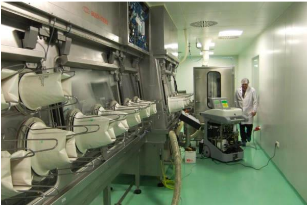
Figure: Isolator connected with VHP Gas generator
